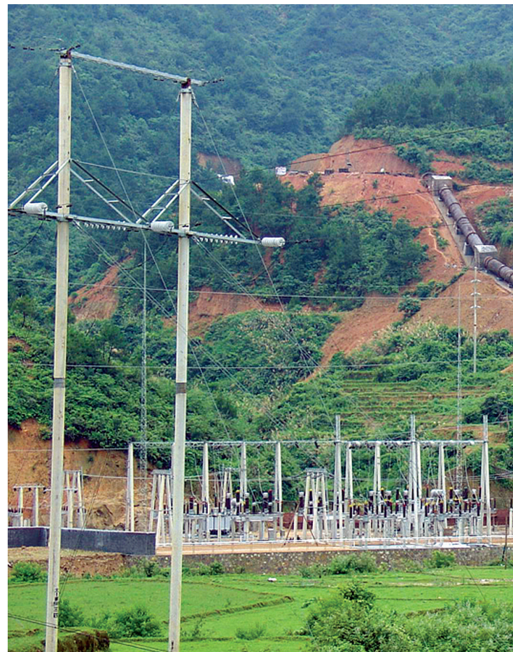
Shimenqiao Small Hydropower Station in Guangxi Zhuang Autonomous Region
